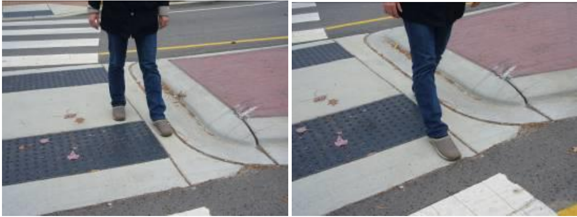
Figure 4-12: Example of Incorrect Detectable Warning Surface installation at a Roundabout crossing
