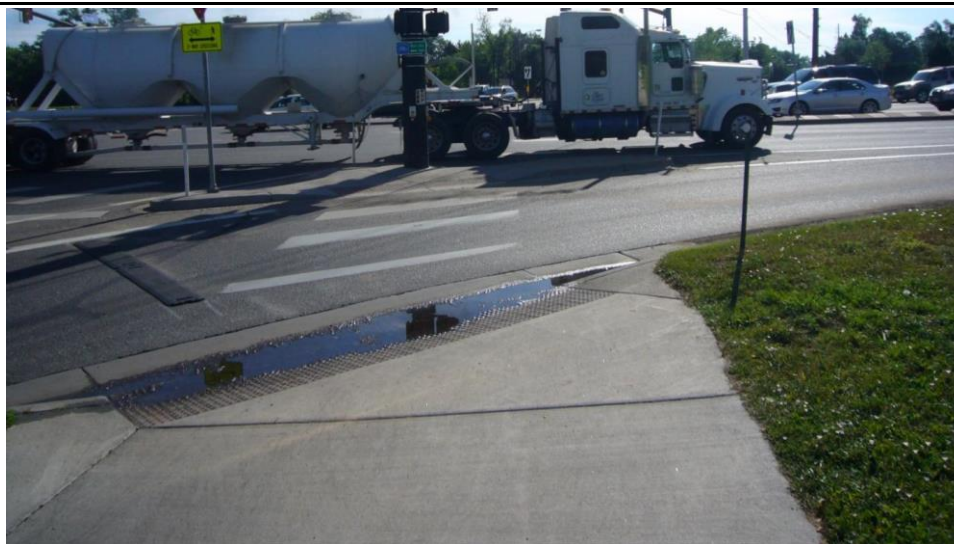
Figure 5-10: Example of poorly aligned crosswalk at CTL
