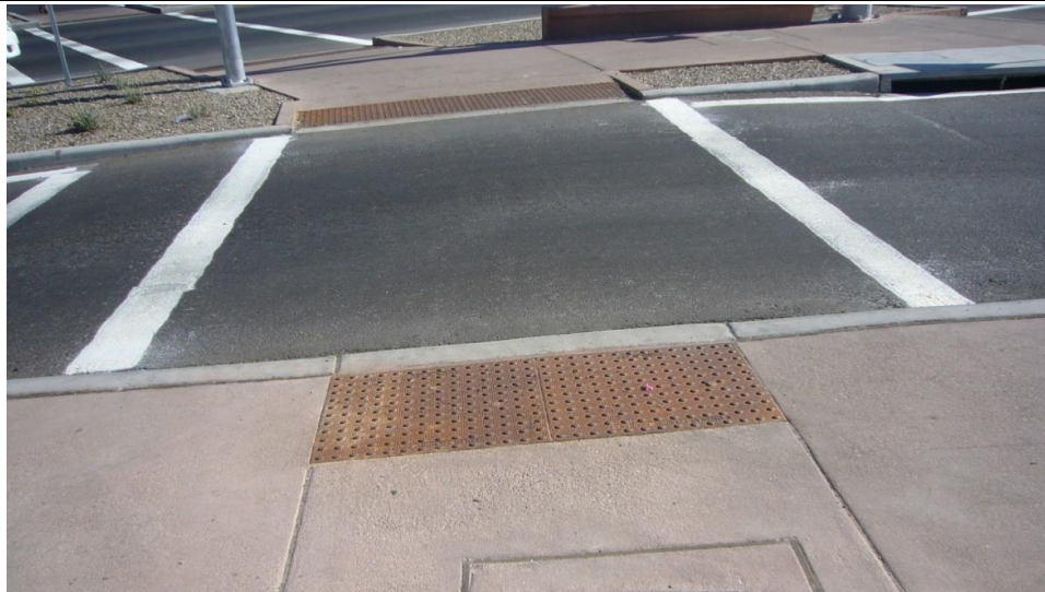
Figure 5-9: Example of properly placed and aligned crosswalk at CTL
