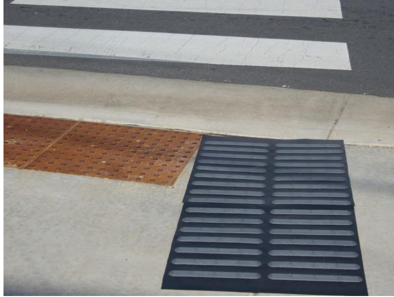
Figure 4-14: Photo of Experimental Bar Tile with bars perpendicular to the crosswalk direction.
