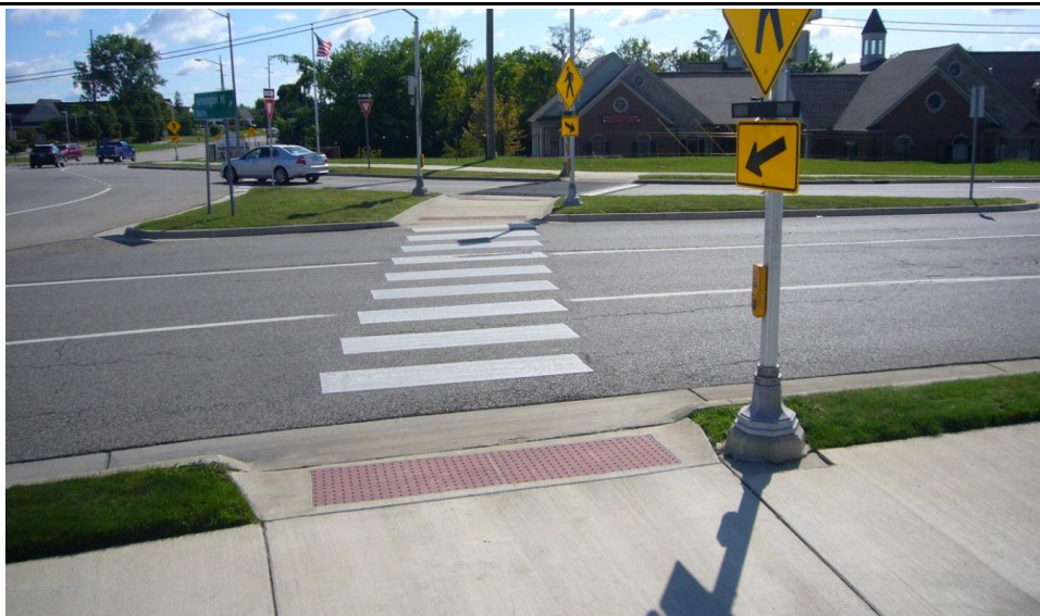
Figure 3-9: Roundabout crosswalk aligned too far to the left of island landing
