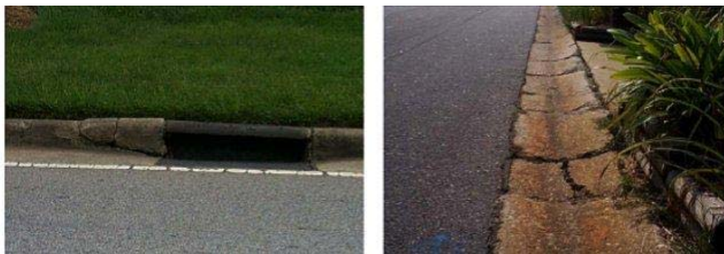
Figure A.5. Gutters damaged.
