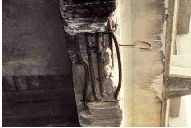
Figure 4.7. Bridge damage due to vertical clearance deficiency collisions.
