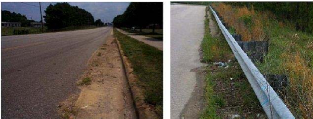
Figure A.4. Gutters blocked.
