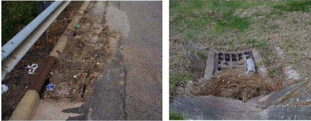
Figure A.6. Inlets blocked.
