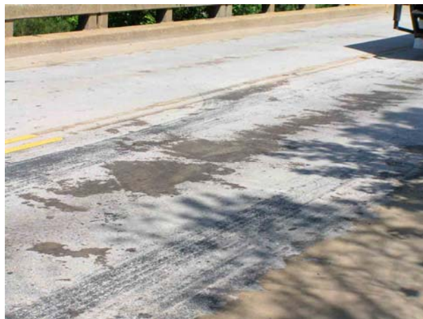
Figure 4.3. Patched concrete deck of bridge.
