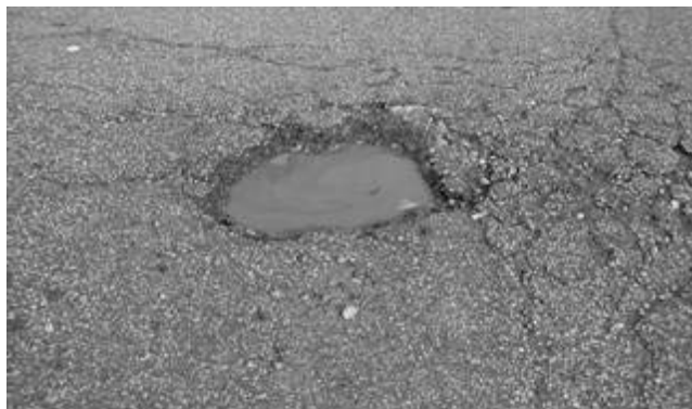
FIGURE B5 Untreated pothole collects water and accelerates pavement deterioration.
