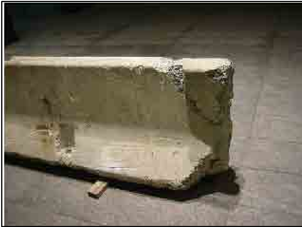
Exhibit 21: Damaged Concrete Barrier
