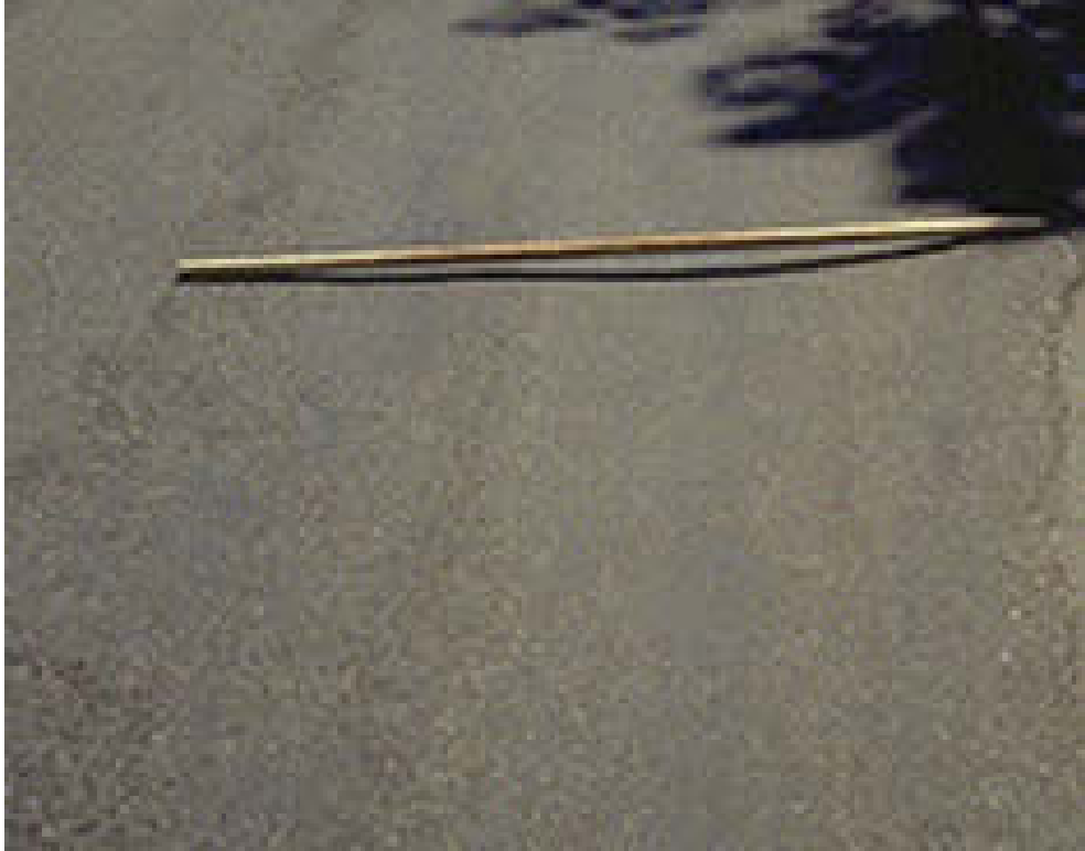
Exhibit 1: Paved Shoulders - Rutting
