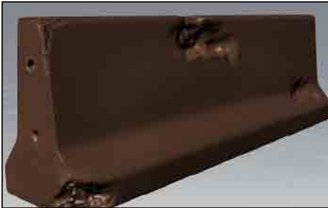
Exhibit 22: Damaged Concrete Barrier
