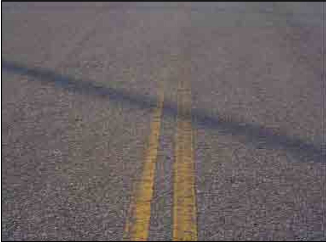
Exhibit 39: Faded Pavement Marking – Center Line
