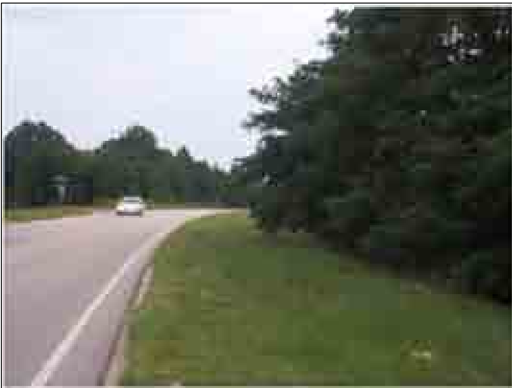
Exhibit 16: Brush & Tree Control – Clear Zone Obstruction
