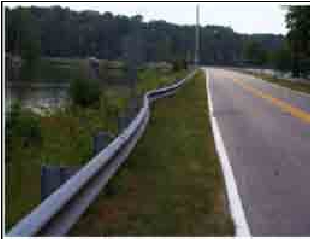
Exhibit 23: Damaged W-Beam Guardrail
