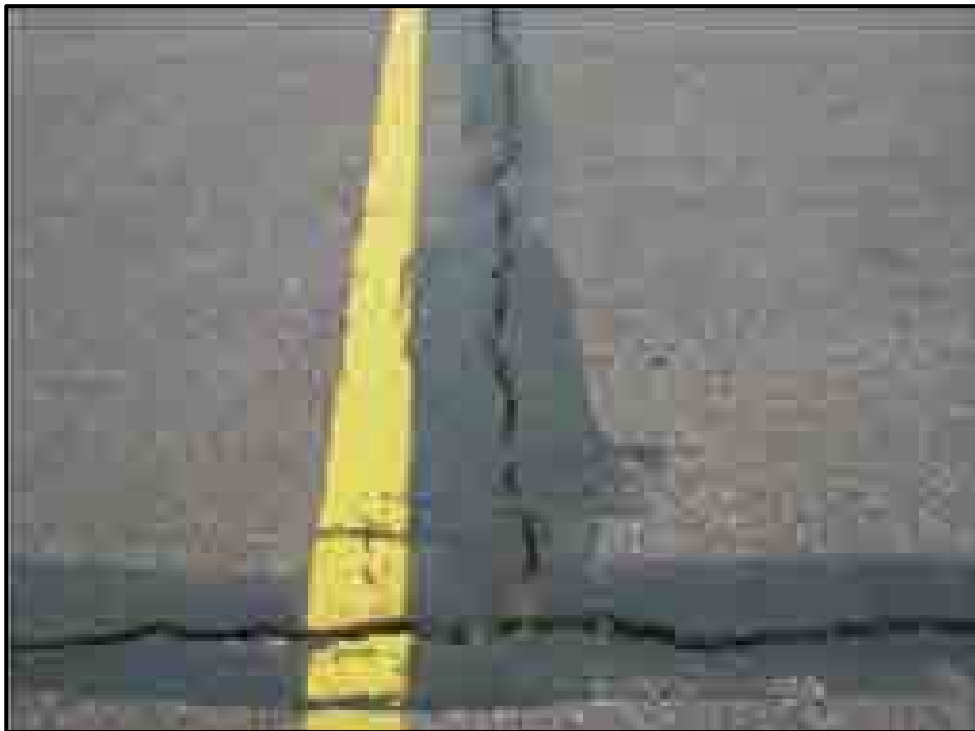
Exhibit 26: Cracked Asphalt Pavement
