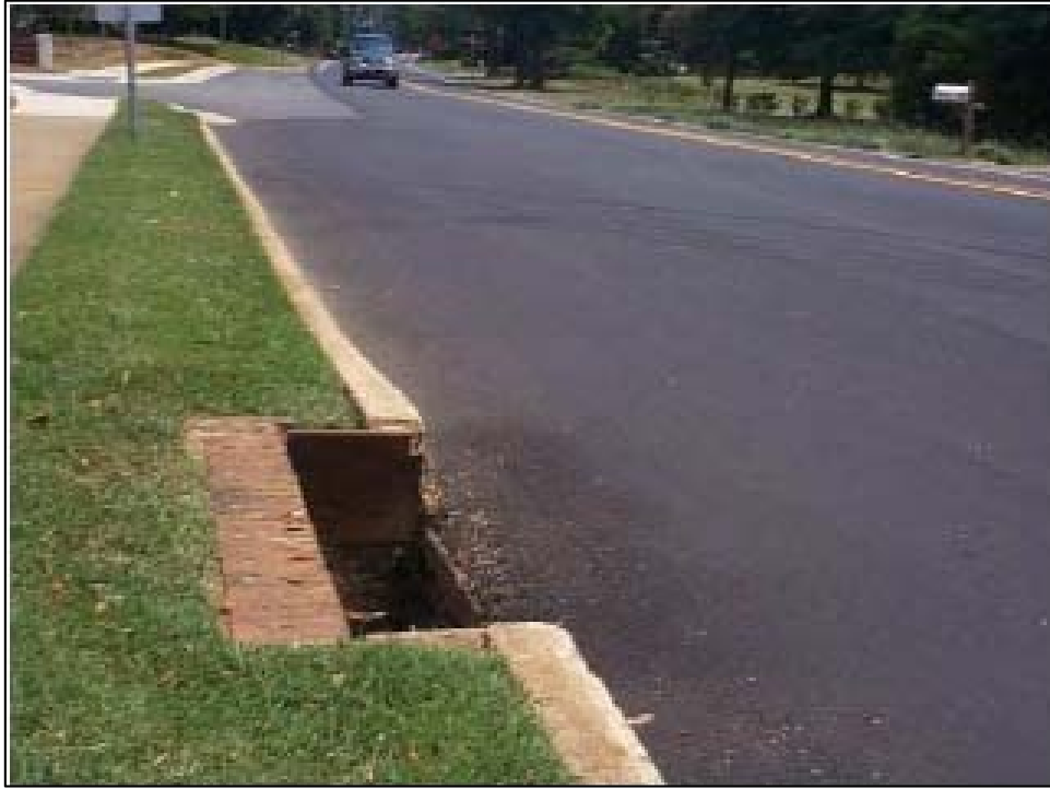
Exhibit 47: Inlet Damaged/Other: Missing
