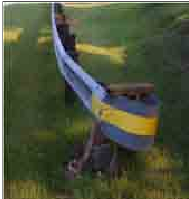
Exhibit 49: Damaged End Treatment
