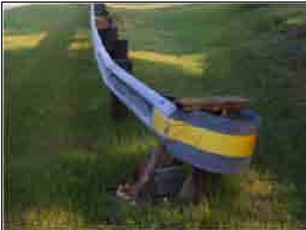
Exhibit 24: Damaged W-Beam Guardrail
