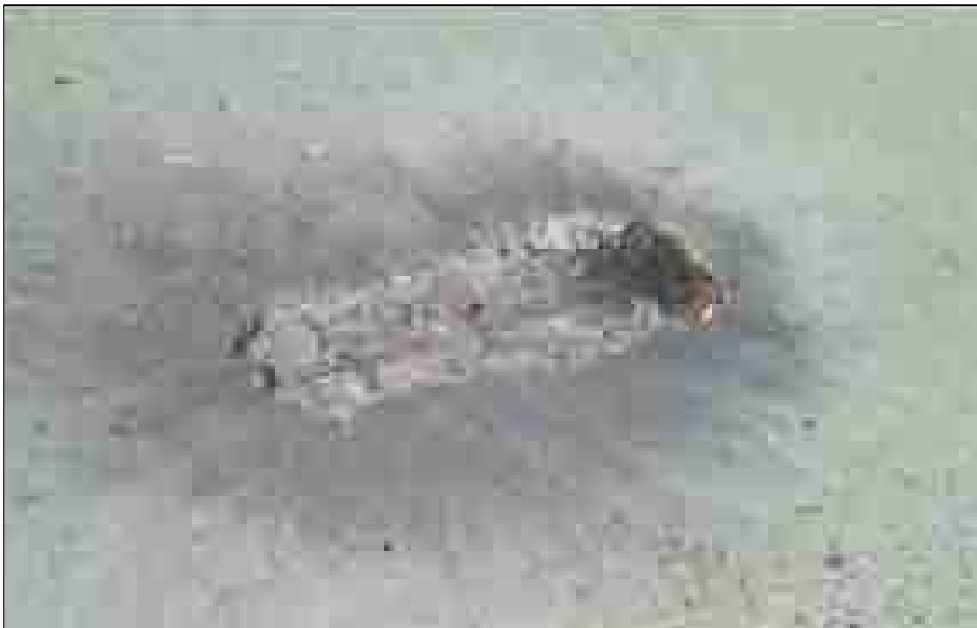
Exhibit 28: Concrete Pavement Spall
